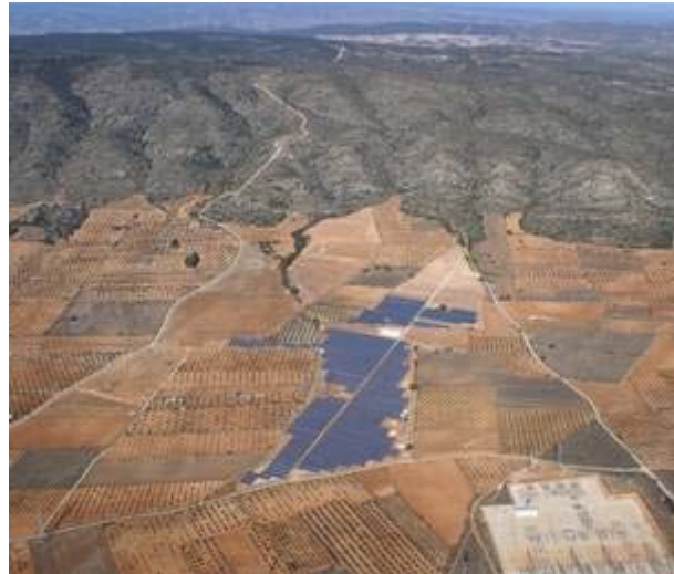
Air view of the construction works in Beneixama in January 2007. The solar park will supply with solar energy to more than 12.000 homes.
